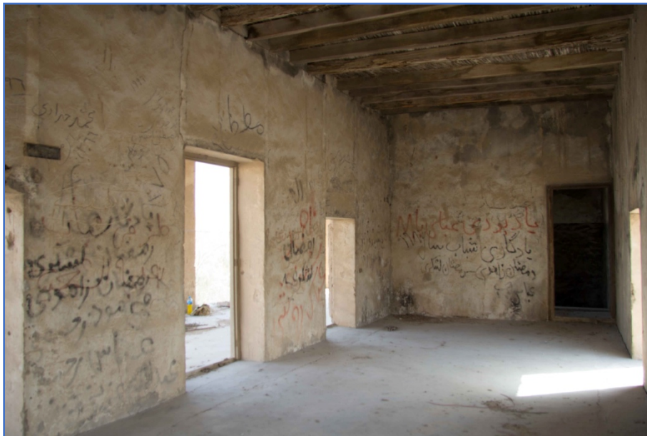
Figure 37: Internal view of Room 1, the door in the far wall opens into Room 2.
