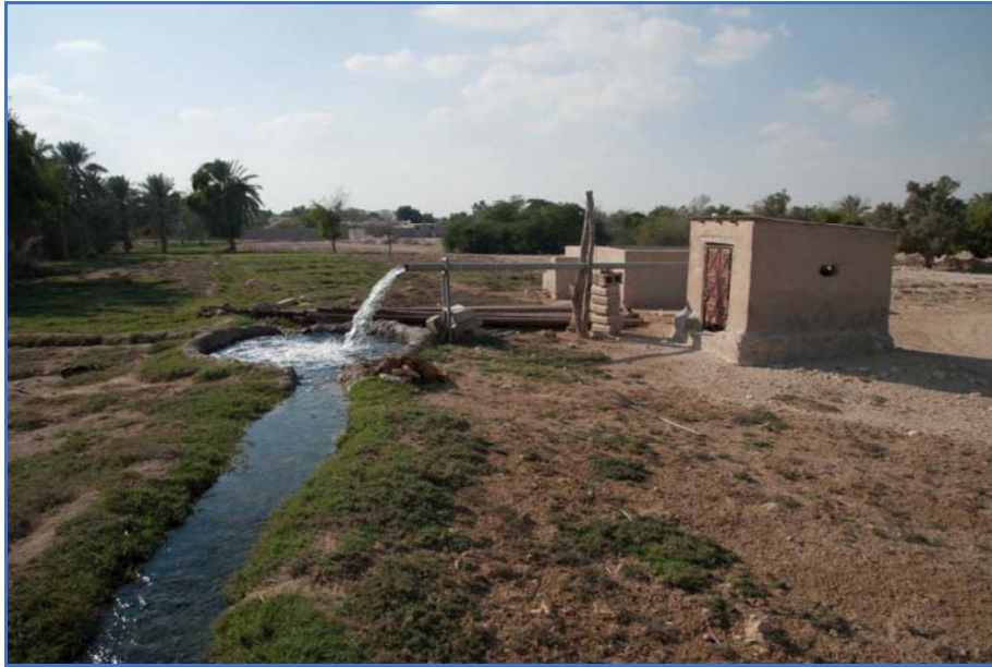
Figure 99: Modern electric pumps extracting water from the lower freshwater aquifer in Rayyan in 2013. The fields are still irrigate using small canals in a traditional manner.
