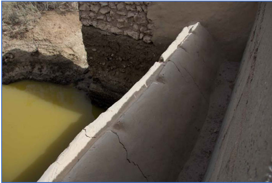
Figure 15 : Trough to catch the water at the top of the well.
