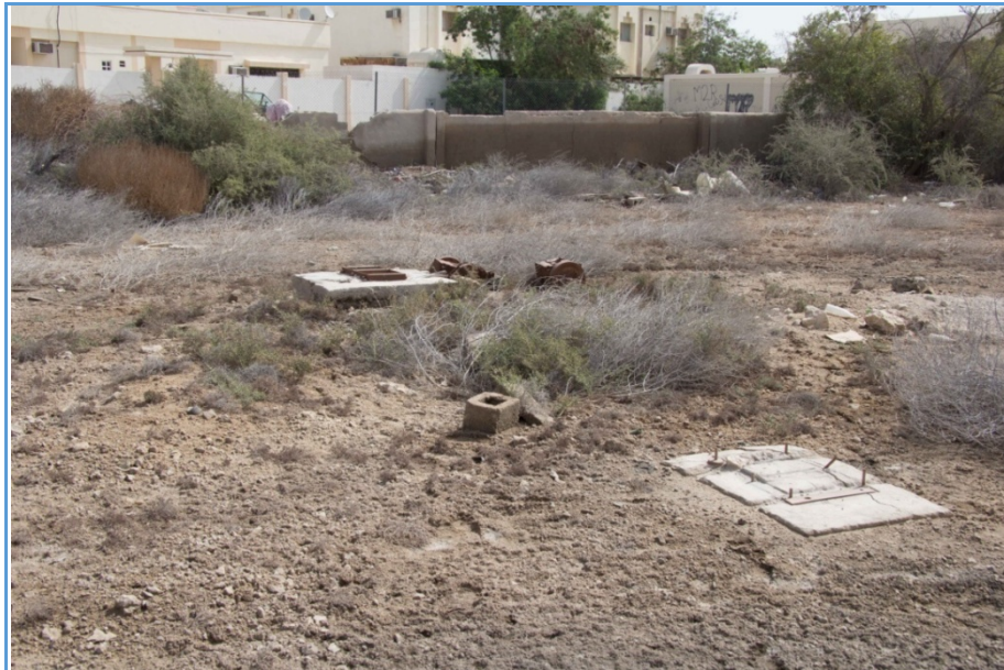
Figure 86: Pump bases Structure 13, with discarded pumps visible behind, looking southeast.
