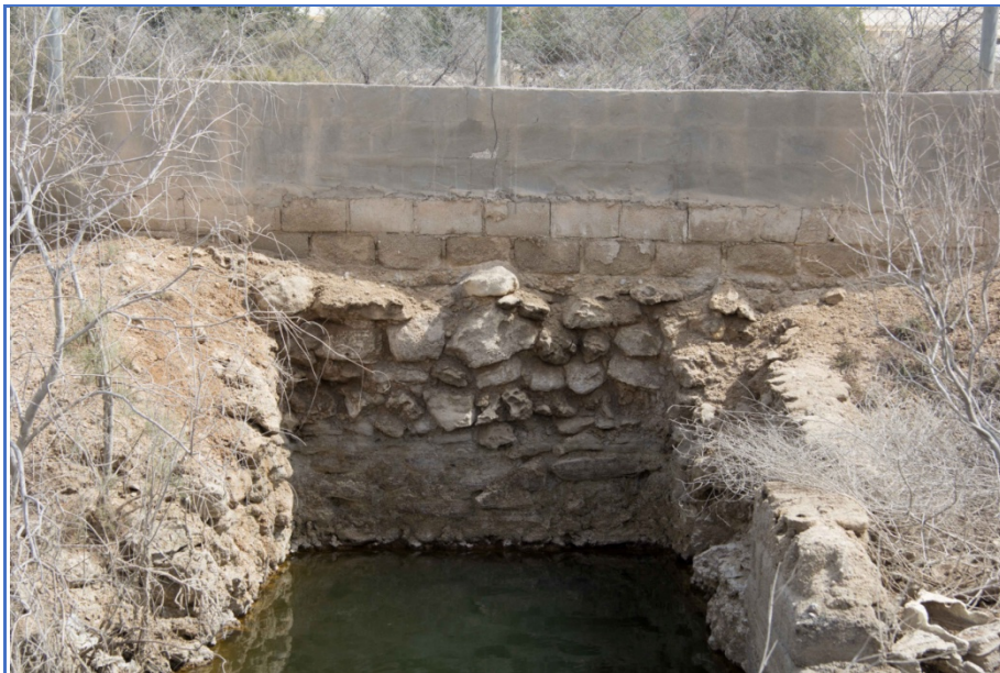
Figure 83: Earlier stone well lining, below later concrete additions associated with Structure 12, looking east.
