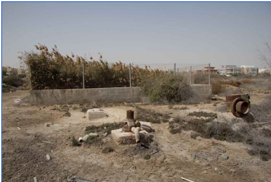
Figure 79: Pump setting in foreground with enclosed overgrown well behind, Structure 10, looking west.
