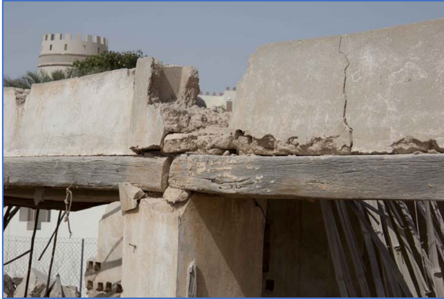
Figure 57: Structural beams, resting on a pillar, over the open end of a stall.
