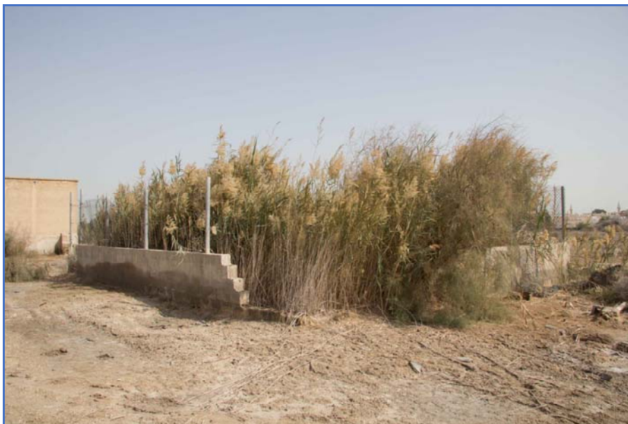
Figure 76: Partially collapsed wall, enclosing overgrown well, Structure 9, looking north.
