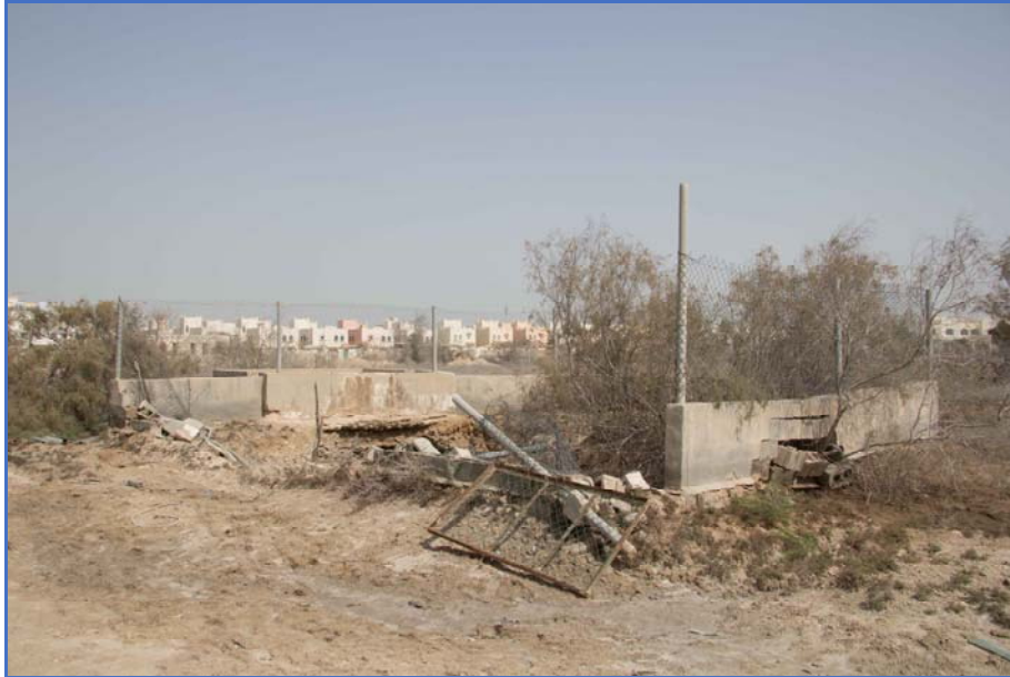
Figure 73: Partially collapsed modern wall and fence around well, Structure 8.
