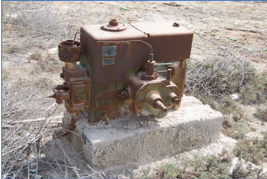
Figure 80: In-situ pump associated with Structure 10.
