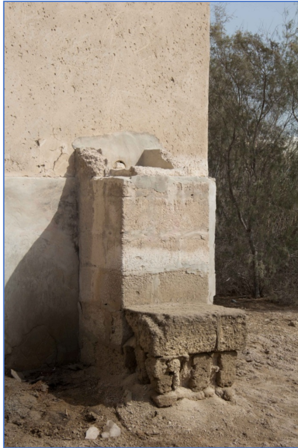
Figure 39: External small trough with a pipe feeding through the wall and into the bath in Room 2.
