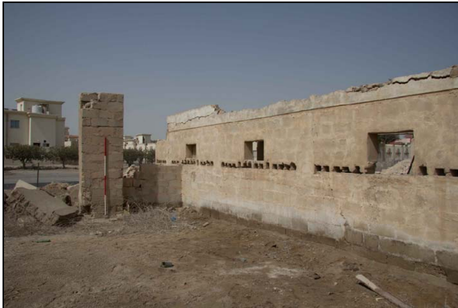
Figure 44: The south side of Structure 3 and the water tank support, looking northwest
