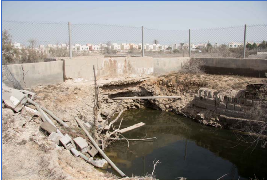
Figure 71: Partially infilled well, Structure 8. Note older stone lining to well visible in places.
